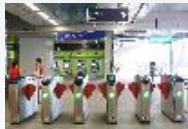
Automatic Fare Collection System
